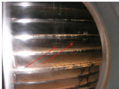
Picture C / damaged kieselguhr cake after emptying
