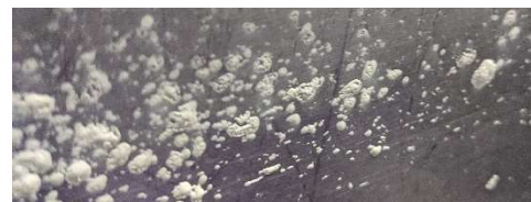
Chlorobutyl close-up on reservoir tank
