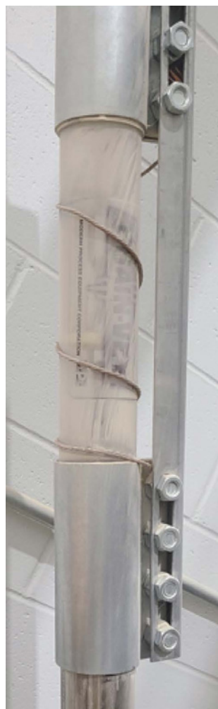
Grounding Wire Jumper
